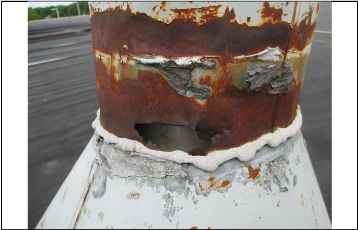
Photo 7: View the asbestos flashing on the north side round vent.
