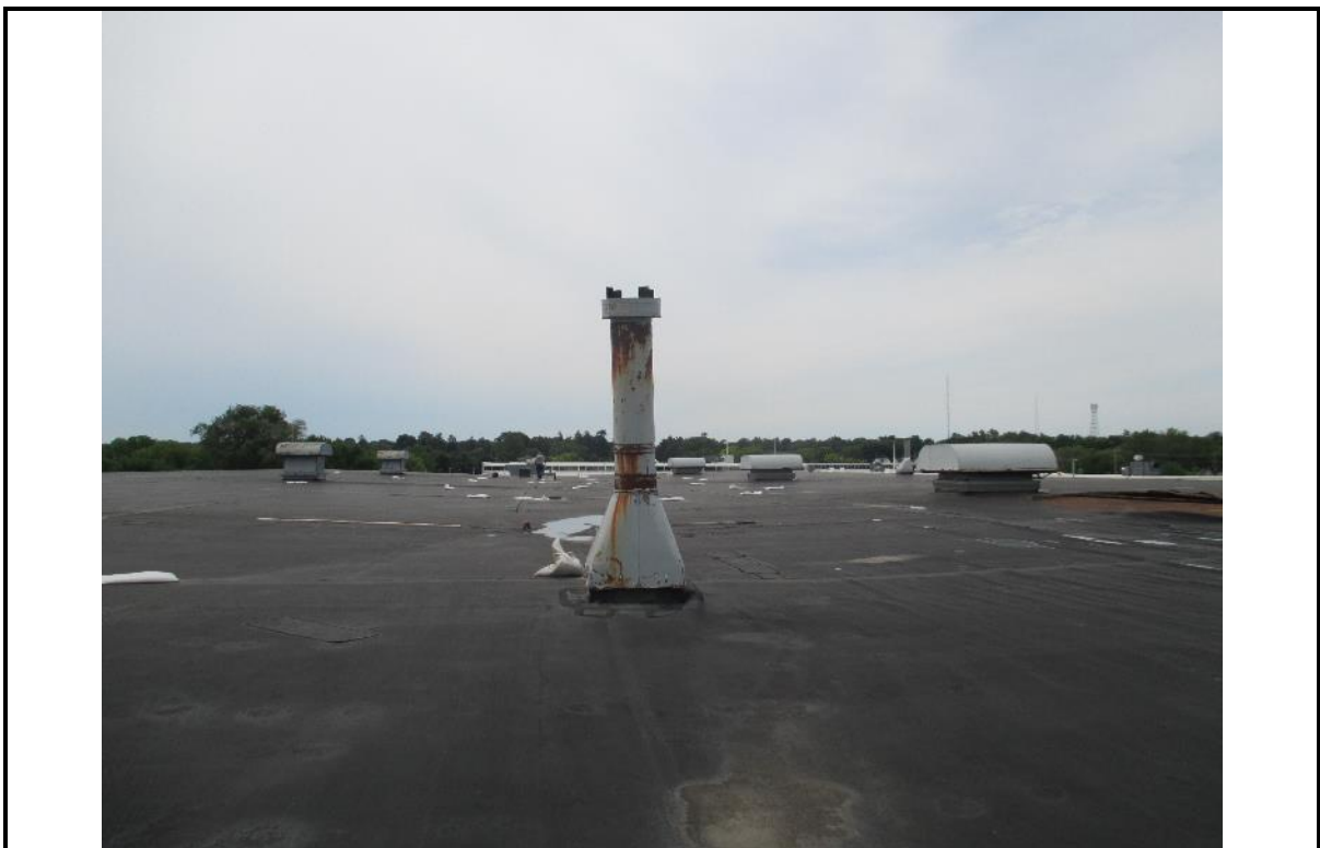
Photo 6: Picture showing the asbestos-containing flashing on the round vent on the north side of the upper roof.
