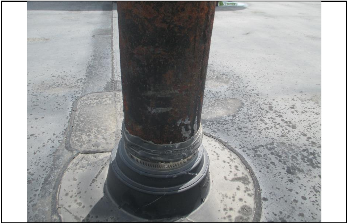
Photo 3: View of asbestos-containing flashing on cast vent on lower roof.
