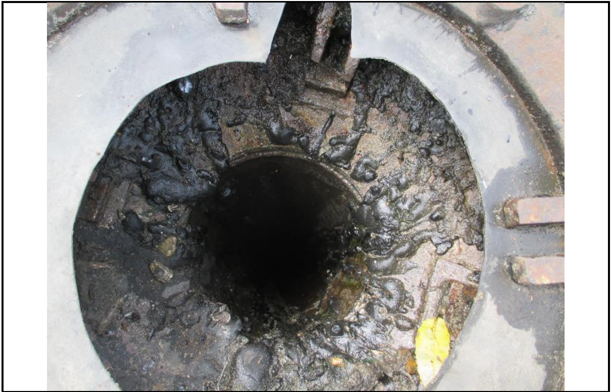
Photo 9: View of the asbestos bituminous coating in the roof drain
